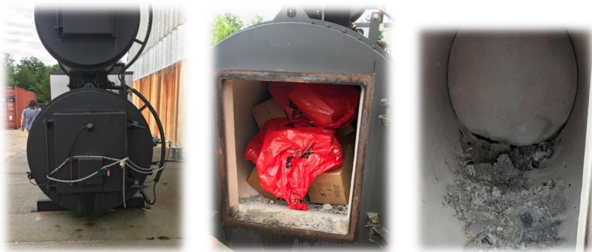
Incinerator used to destroy illegal drugs/narcotics, maintained and operated by TBI personnel.
